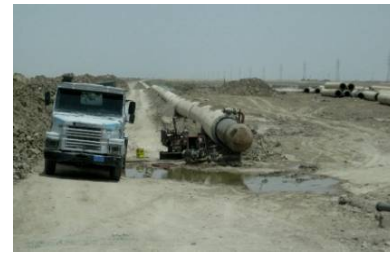
Oil piping networking
